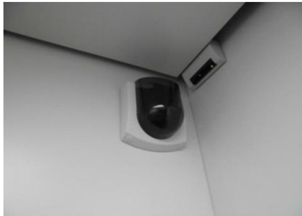
Photo11 : Security camera installed in an elevator
