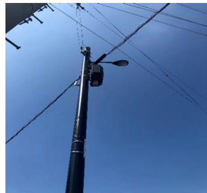
Photo6 : Security light installed
